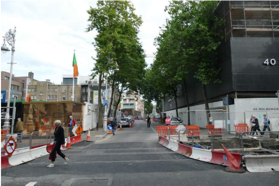
Molesworth Street, Dublin, September 2016. Canada House (built 1982) and the Passport Office (built 1975) have been demolished. Photo Colm Murray.
